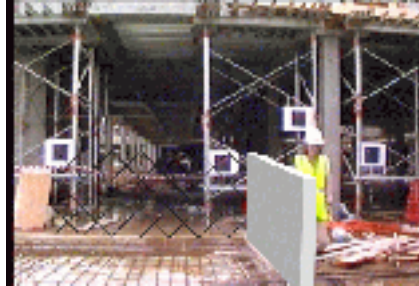
Figure 6: Outdoor construction site, augmented with a virtual wall about to be built
